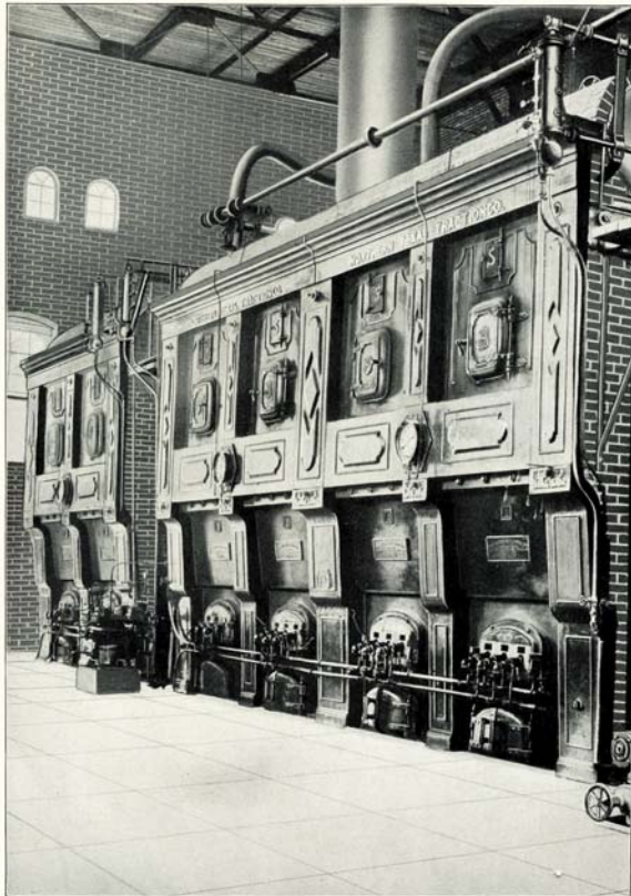
STIRLING BOILERS ARRANGED FOR BURNING OIL
